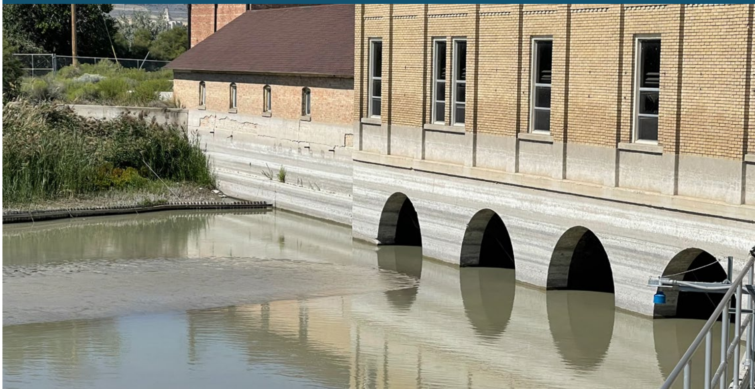
Utah Lake Outlet Pump Station Water Level Lines Reflect Drought - A. Kimmerle
