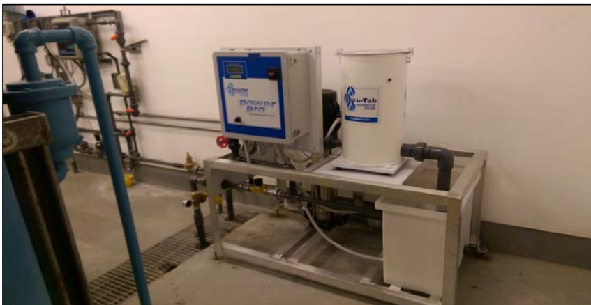
Installed skid-mounted chlorinator 1526 East 8600 South
