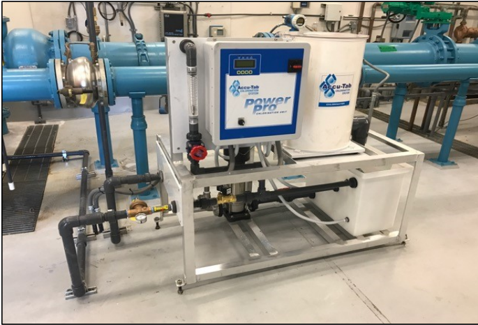
Installed skid-mounted chlorinator 968 East 8520 South
