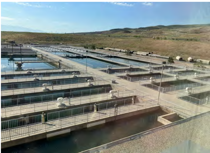
Inclined plate settlers installed and functioning in basins 5 and 6
