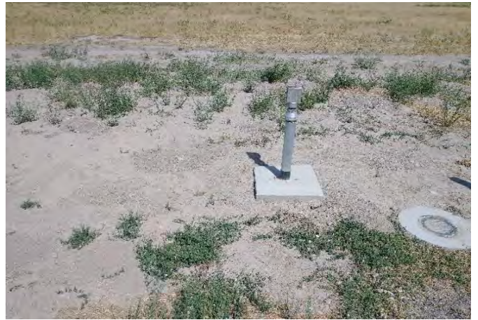
New test station
