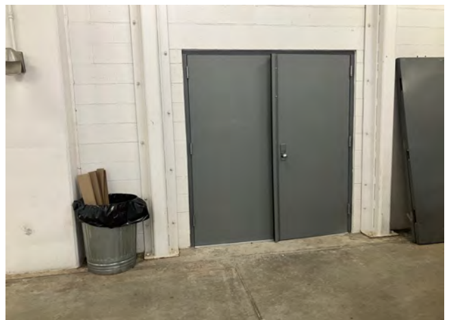
Installed acoustical door
