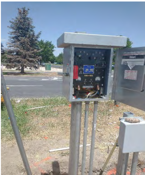
New cathodic rectifier
