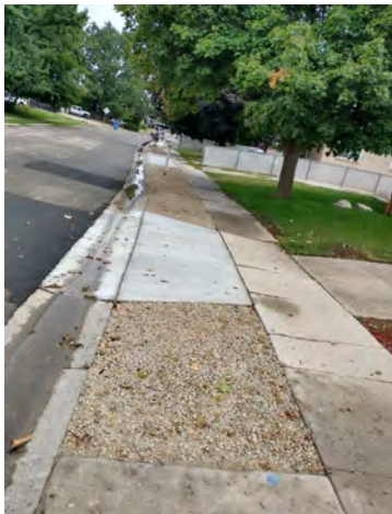
New driveway approaches and park strips over new pipeline on Redmaple Dr.
