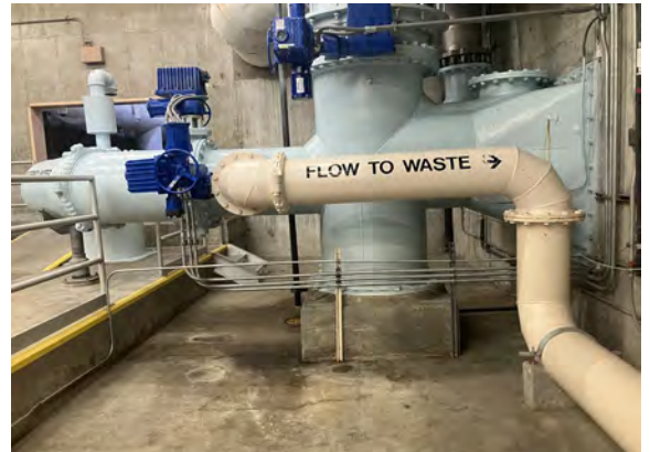
Existing Filter to Waste Piping
