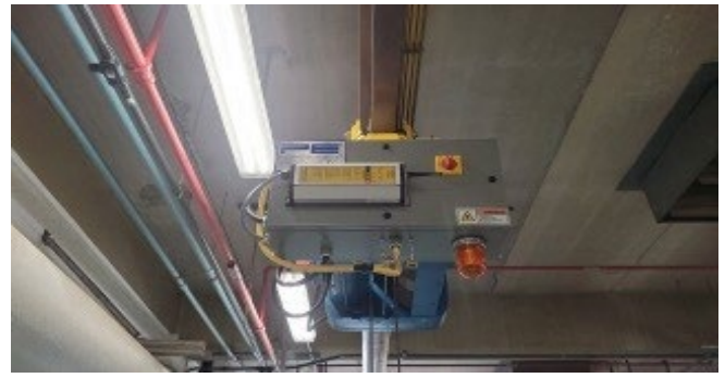
New crane controls (gray)
