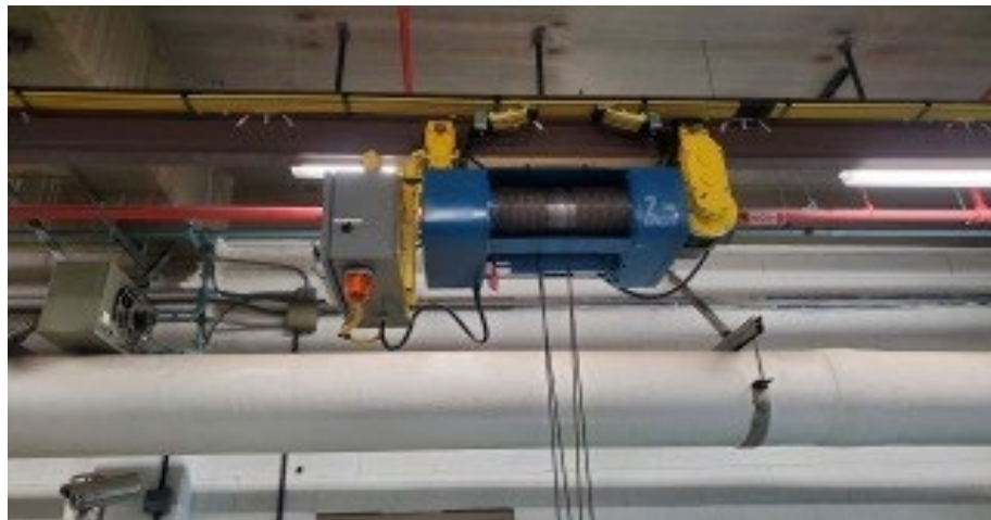
New crane assembly including trolley (yellow), hoist (blue) and controls (gray)
