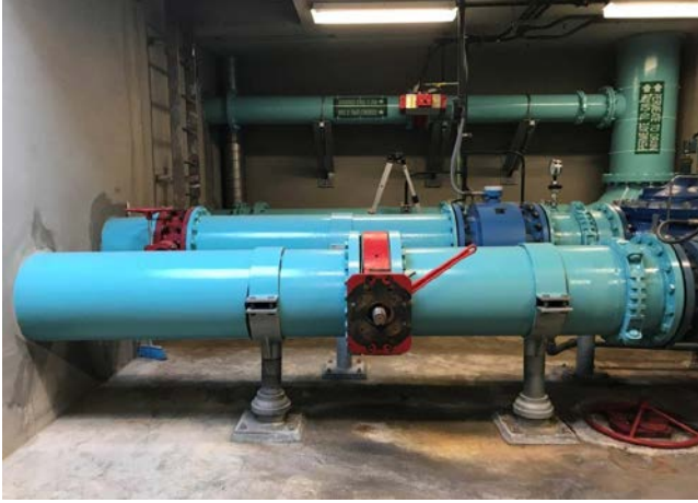
Piping configuration prior to project
