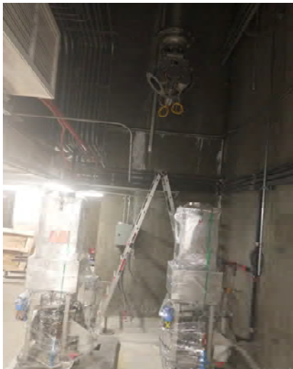
Newly placed wetting systems and wye diverter for polymer system
