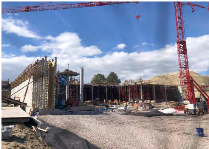
West end of the reservoir being prepared with scaffolding for the installation of the concrete roof deck
