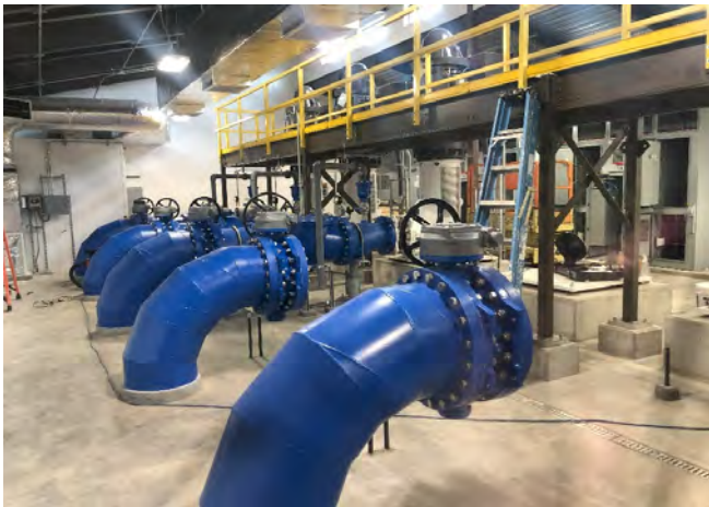
Interior of the new pumpstation
